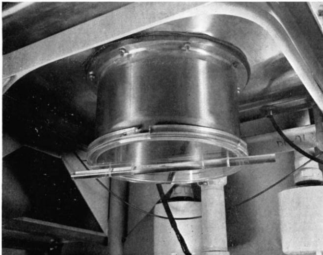
FIG. 10.—Large transfer unit connection.
